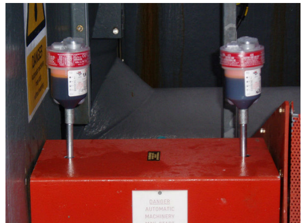
Extraction fan bearing lubrication
