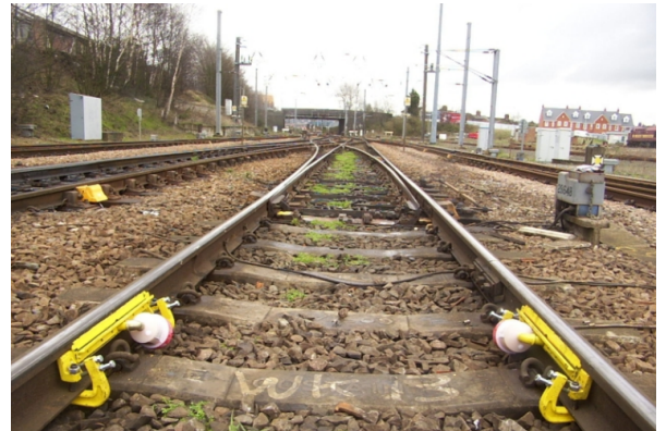
Electro-Lubers™ on rail tracks
