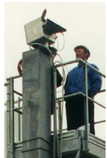
Linescanner in protective housing is mounted on top of a tower.
