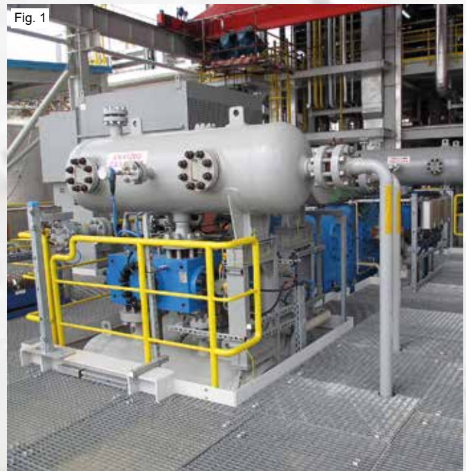
Fig. 1: Installed reciprocating compressor unit
