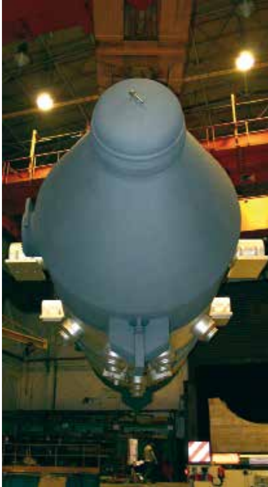
Waste heat boiler
