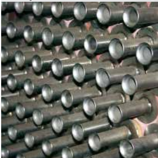
Ferrule at gas inlet tubesheet
