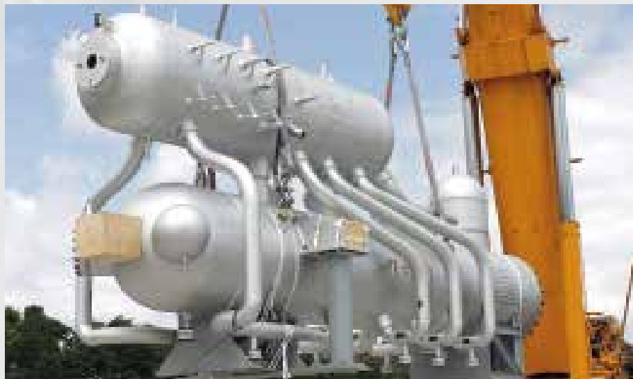
Process gas waste heat recovery system
