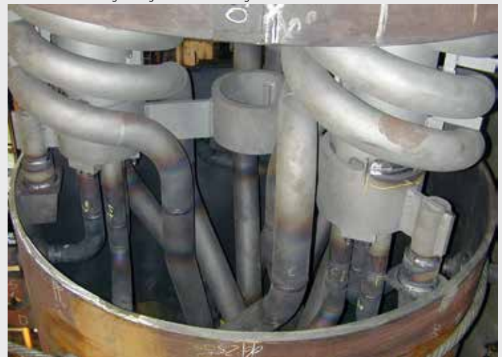
Interconnecting tubing to helical heating surfaces
