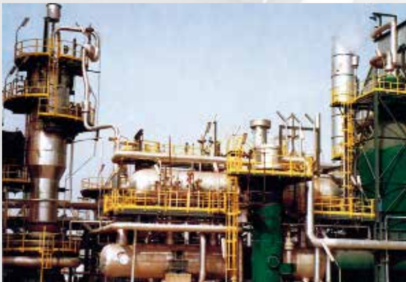
Ammonia plant with synloop WHB, reformed gas WHB, steam superheater and steam drum
