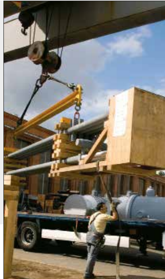
Transfer Line Exchangers at the works area
