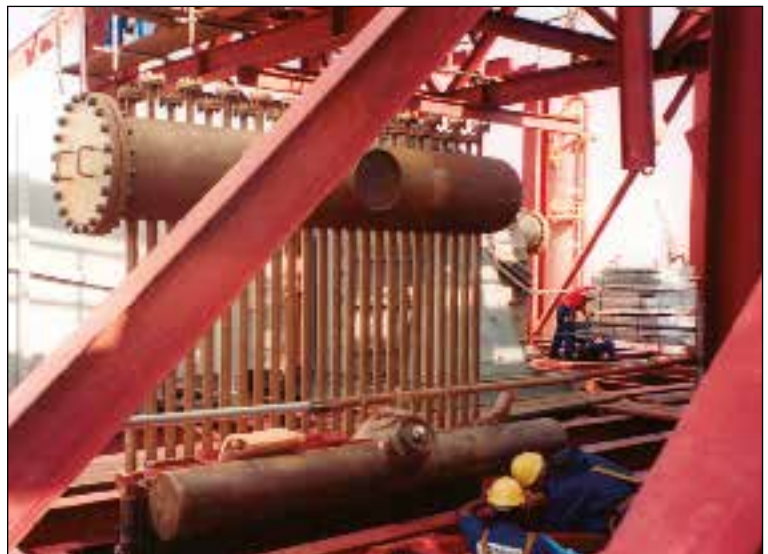
Upper end of BLQ with gas collection head and riser header
