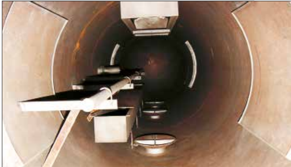
Steam drum internals
