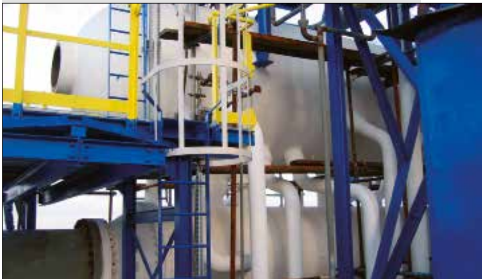
Secondary Transfer Line Exchanger / Steam Drum Unit
